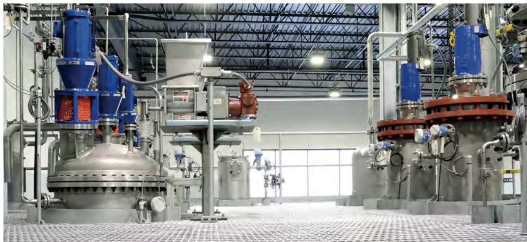
The pilot plant
