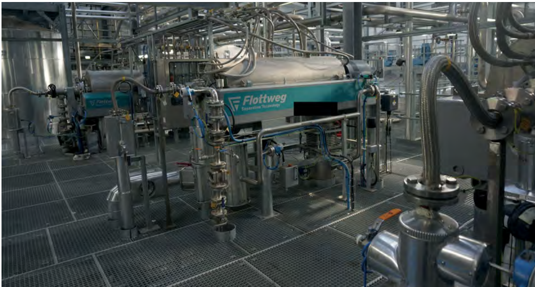
A Tricanter Pretreatment plant
